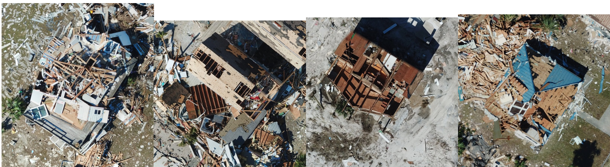
Figure 9. Example buildings labeled 'major damage'.
